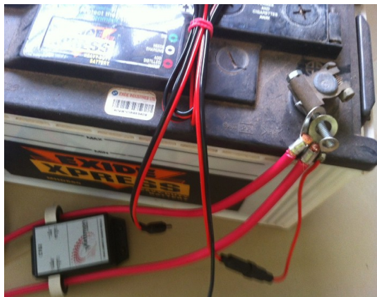
Figure 1.5 Positive battery terminal connection
